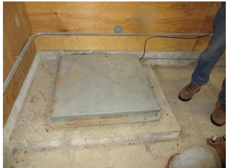
Photograph 10: Storage tank hatch inside pump house
