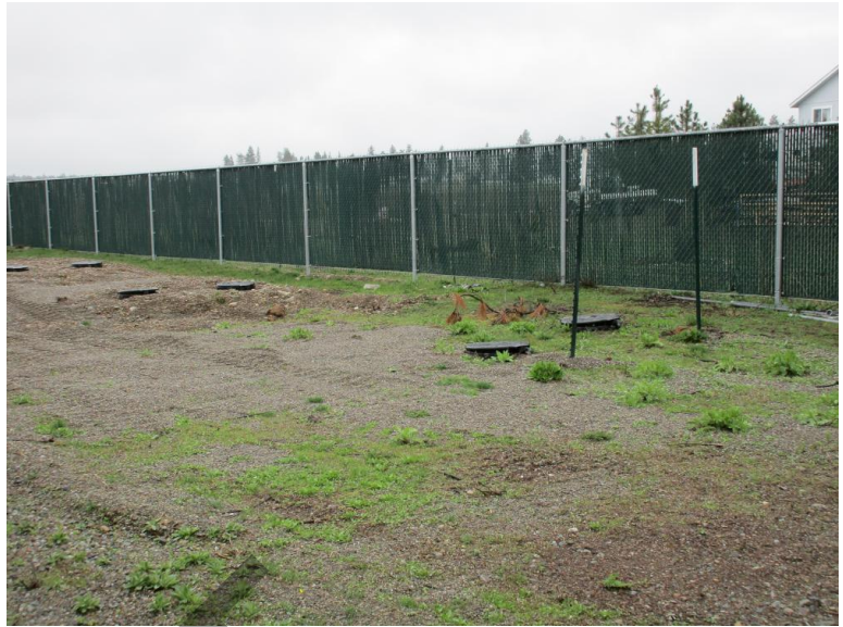
Photograph 2: Six underground propane tanks - 1000 gallons each
