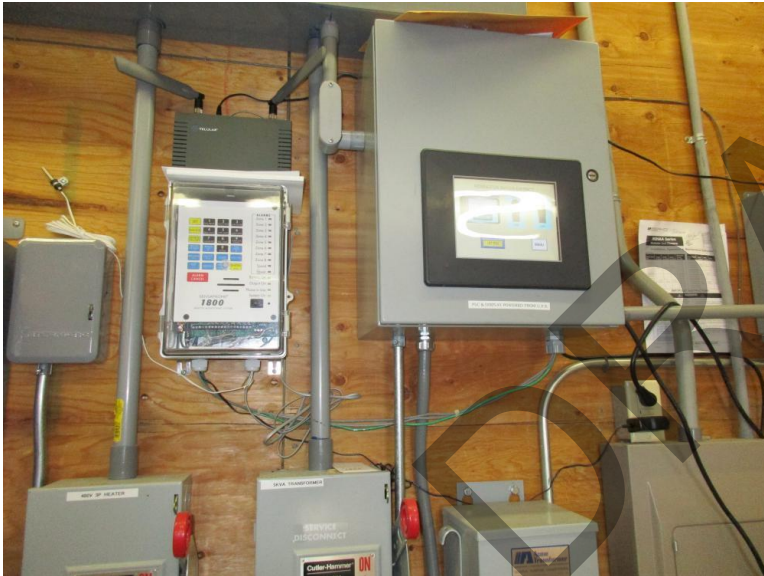
Photograph 17: Control panels, Sensaphone panel for emergency contact
