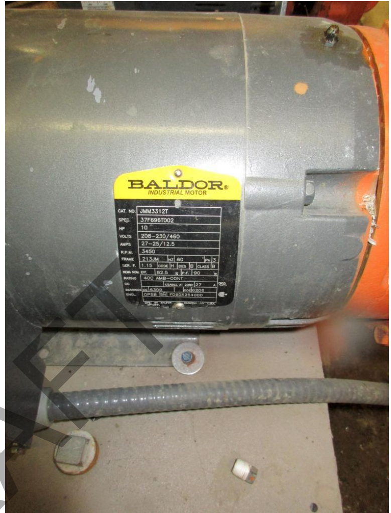
Photograph 8: 10 HP Baldor booster pump
