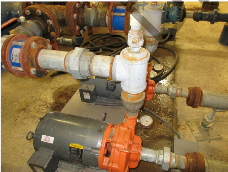
Photograph 9: Two 10 HP booster pumps
