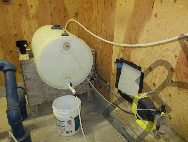
Photograph 13: Sodium hypochlorite injection
