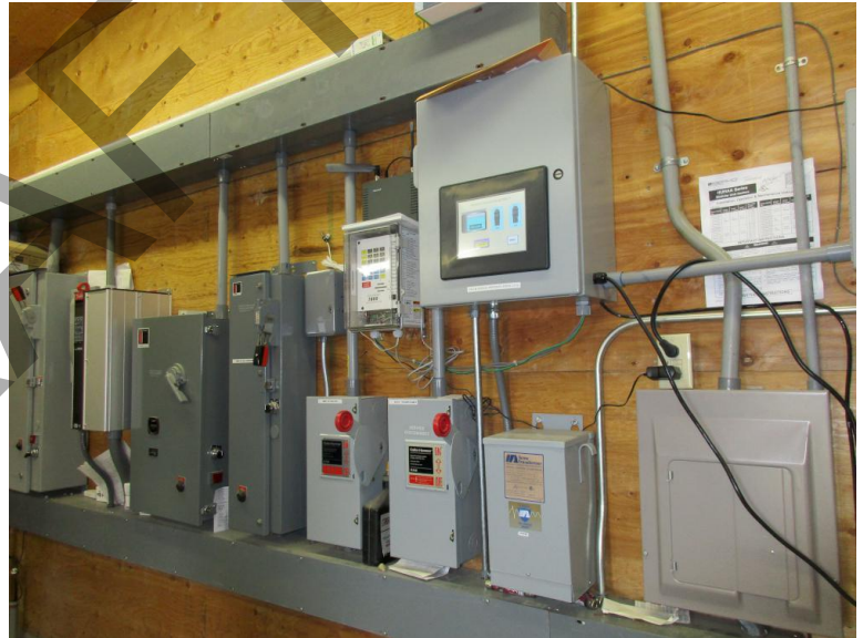
Photograph 18: Control panels inside pump house
