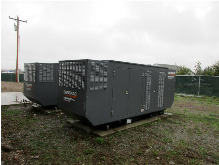
Photograph 1: Two new 150 HP propane powered generators
