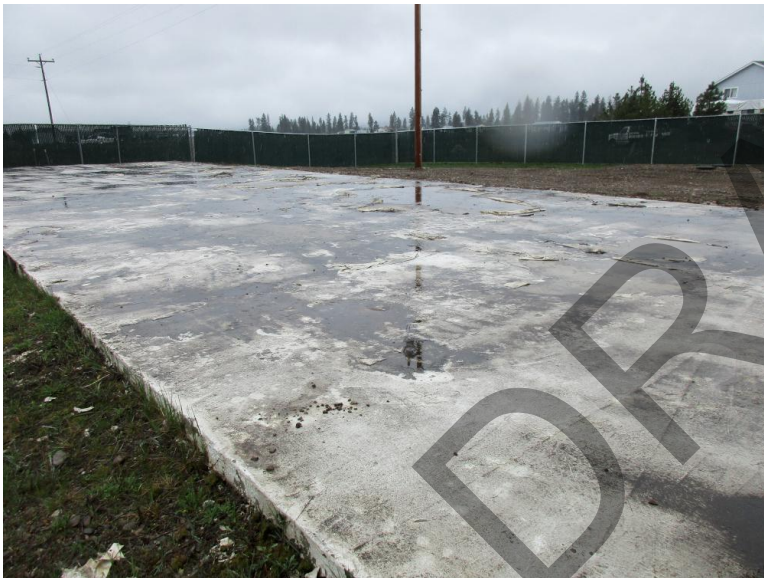
Photograph 3: Storage tank roof showing signs of peeling of sealant
