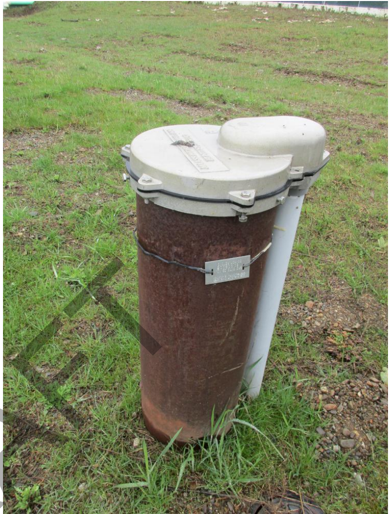
Photograph 20: Well 2 located on the fenced storage tank and pump house lot.
