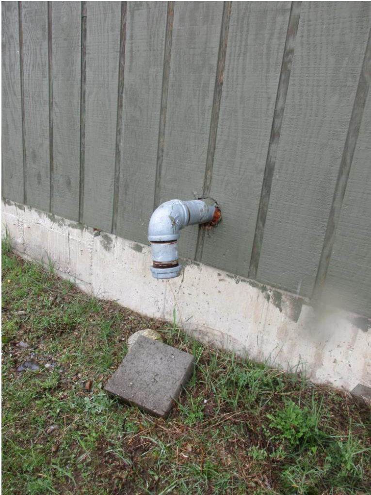
Photograph 5: Flow to waste from pump house.
