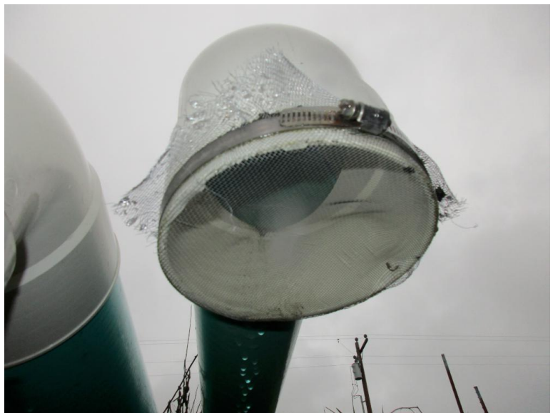
Photograph 22: Screen on reservoir flow to waste
