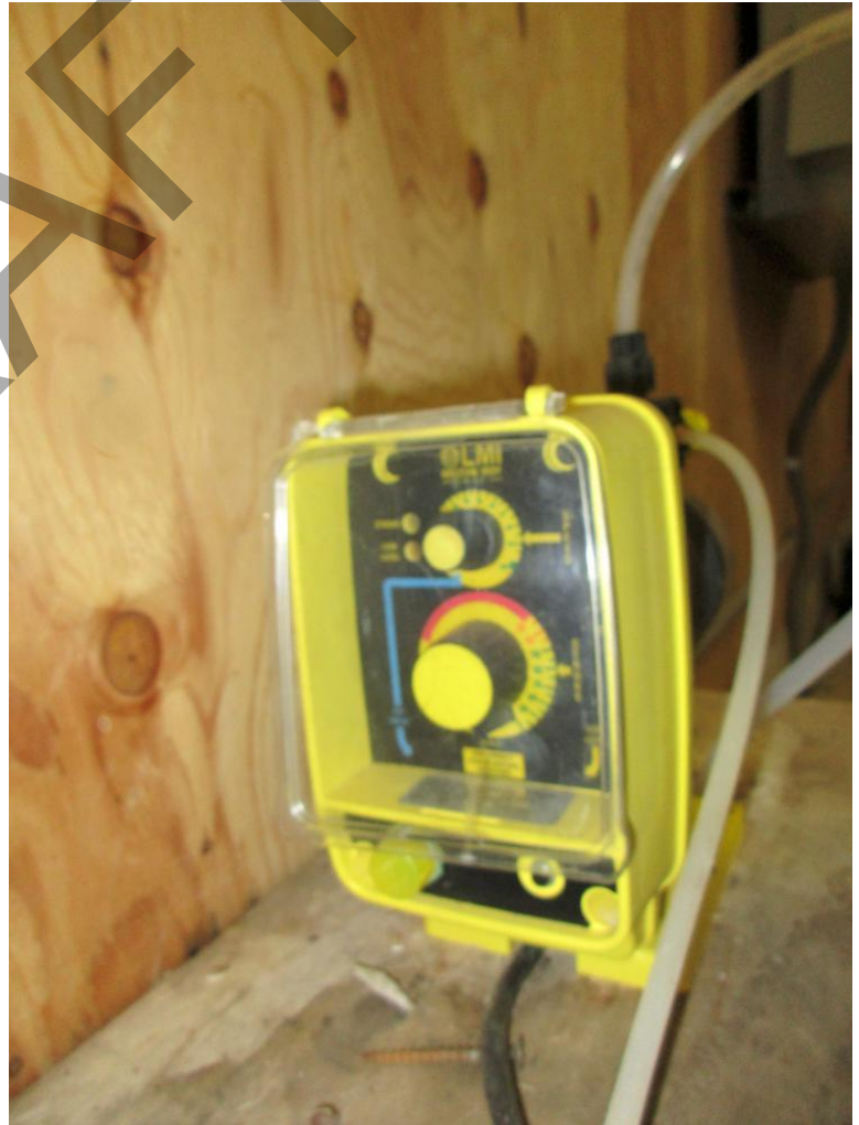
Photograph 14: LMI metering pump
