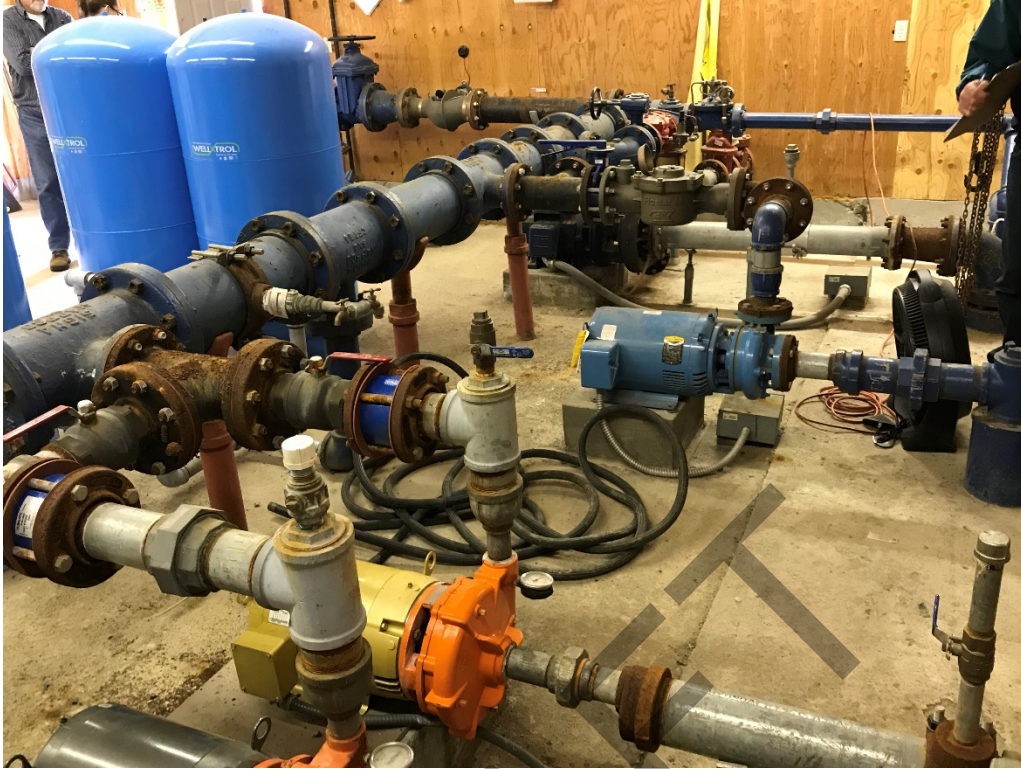
Reservoir with Pump House
