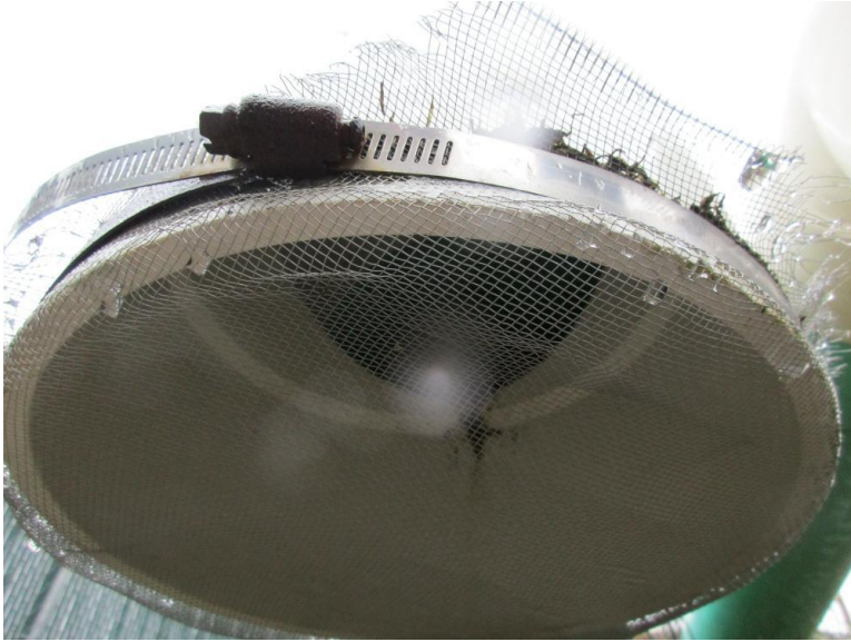
Photograph 23: Screen on storage tank flow to waste
