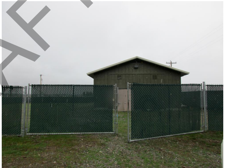
Photograph 26: View of pump house storage tank and well 2 lot
