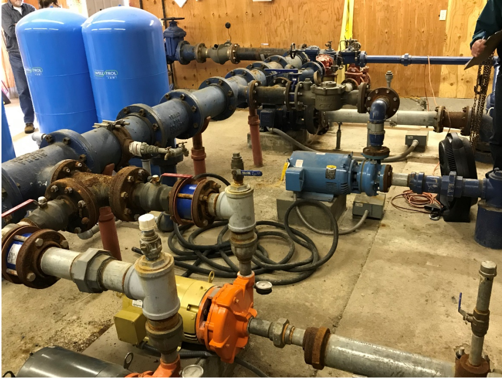
Booster Pumps in Pump House
