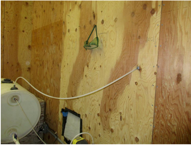
Photograph 15: Chlorine tank vent to outside.
