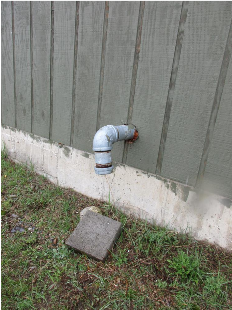
Photograph 5: Flow to waste from pump house.
