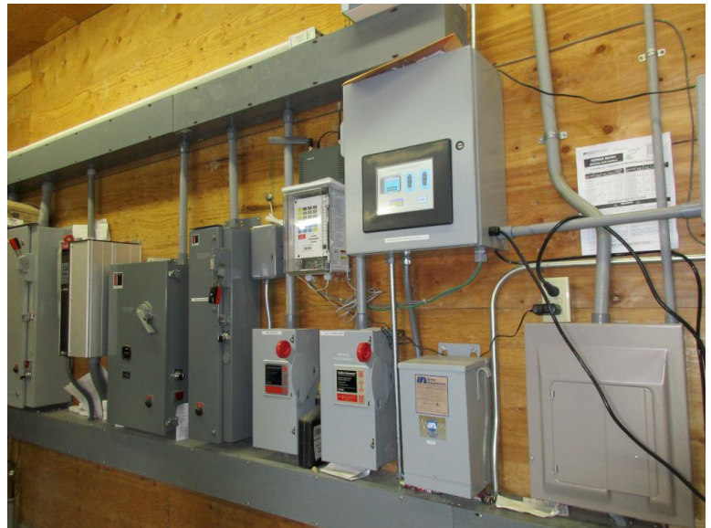
Photograph 18: Control panels inside pump house
