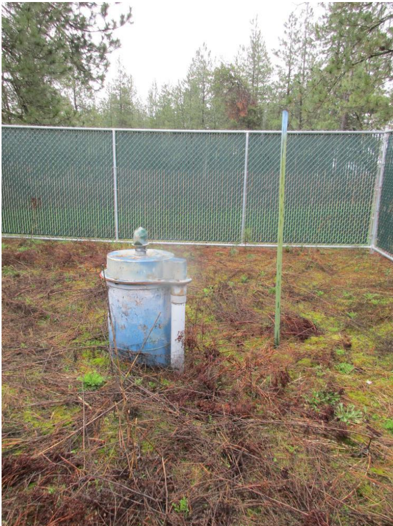
Photograph 25: Well 1 located across street from pump house
