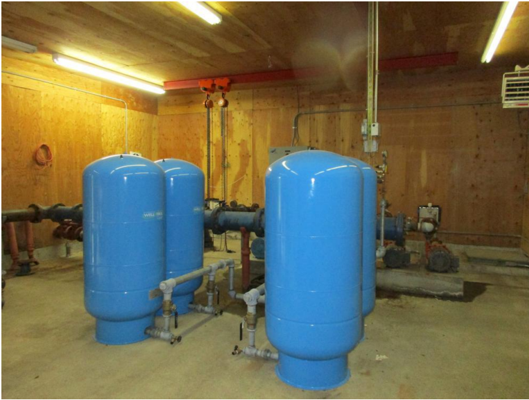
Photograph 7: Four pressure tanks for buffer and back up pressure for system
