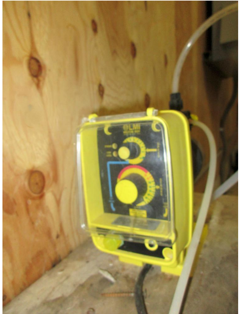
Photograph 14: LMI metering pump
