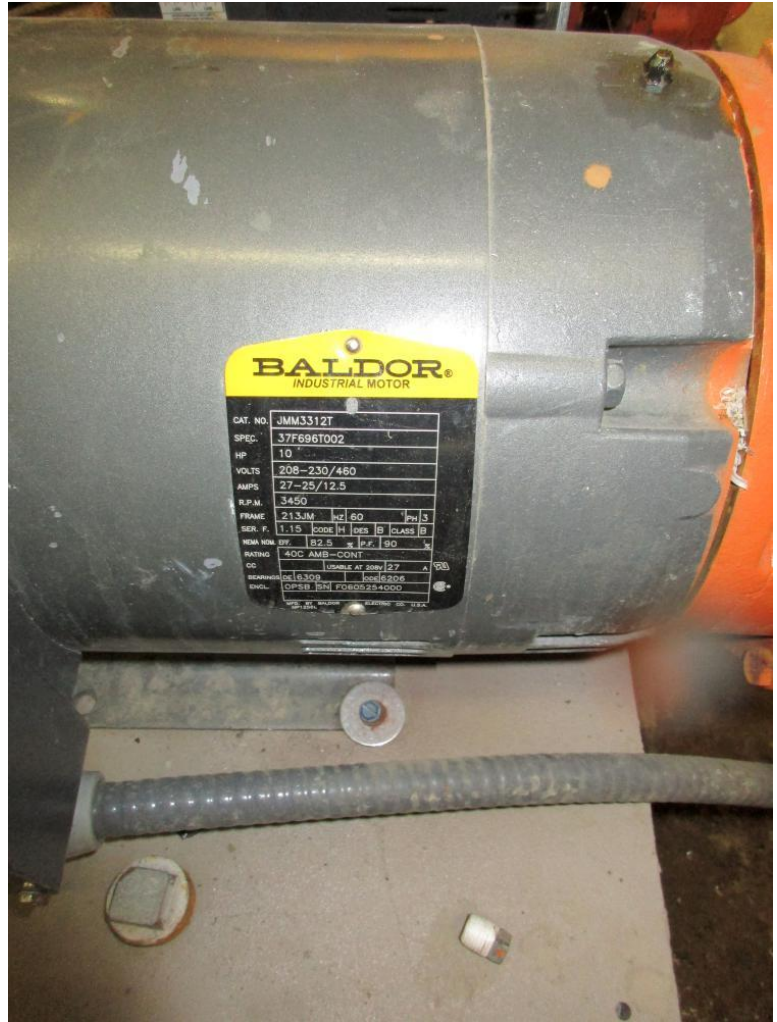
Photograph 8: 10 HP Baldor booster pump
