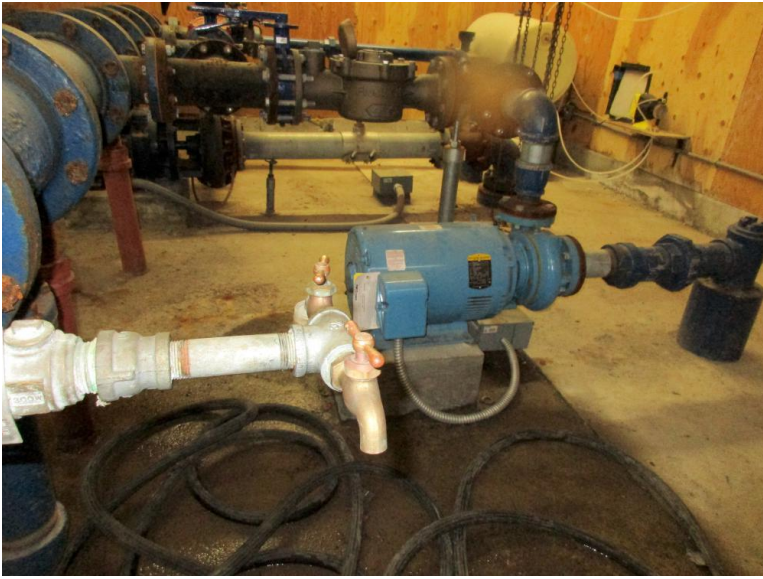
Photograph 11: 20 HP booster pump used during peak summer demand
