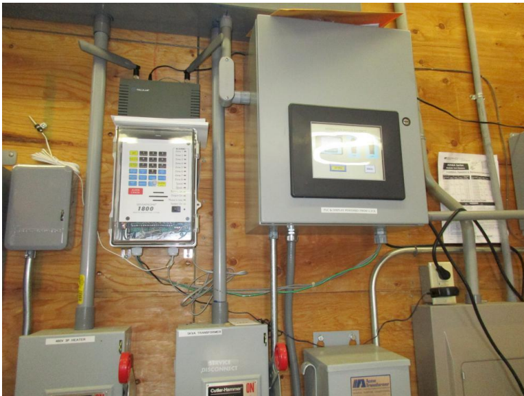
Photograph 17: Control panels, Sensaphone panel for emergency contact
