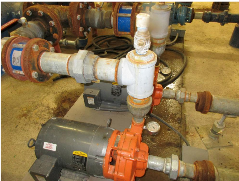
Photograph 9: Two 10 HP booster pumps
