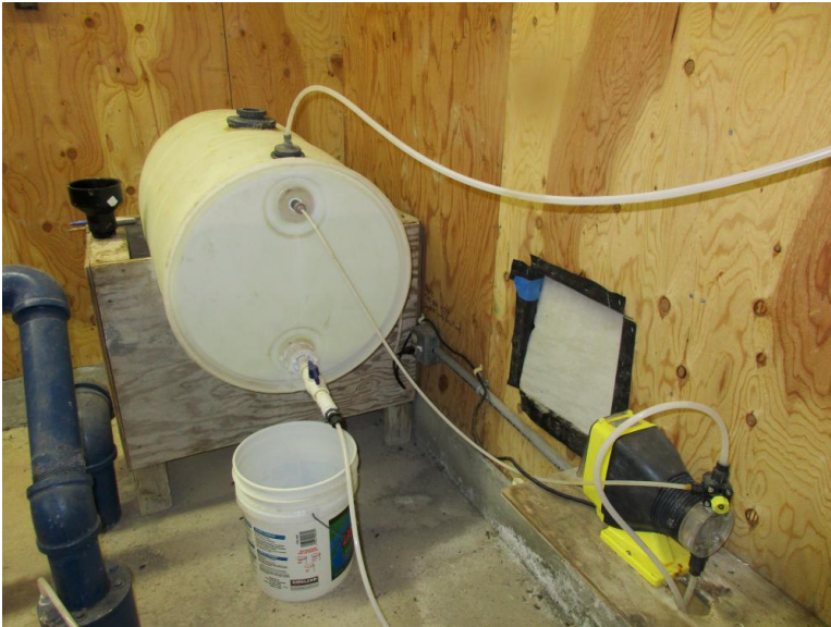
Photograph 13: Sodium hypochlorite injection
