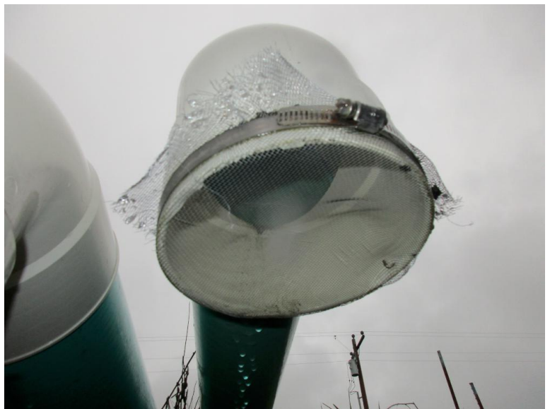
Photograph 22: Screen on reservoir flow to waste
