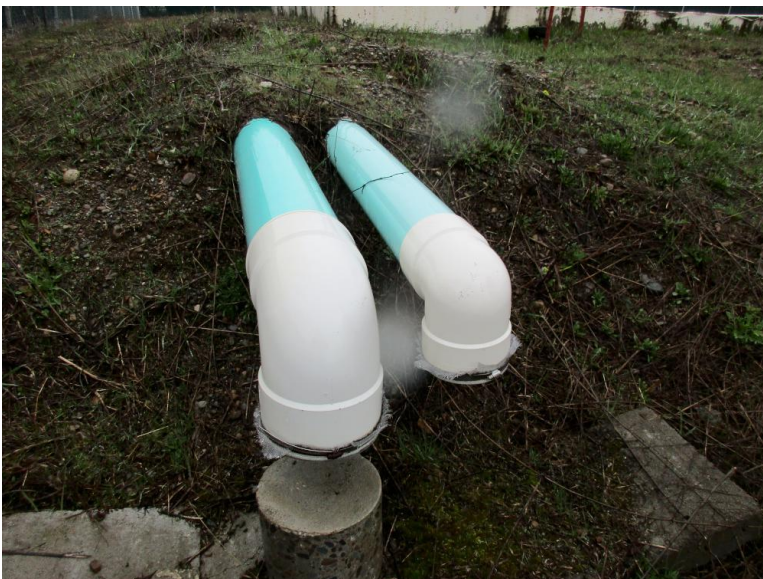
Photograph 21: Overflow-flow to waste for reservoir, screened and splash plate
