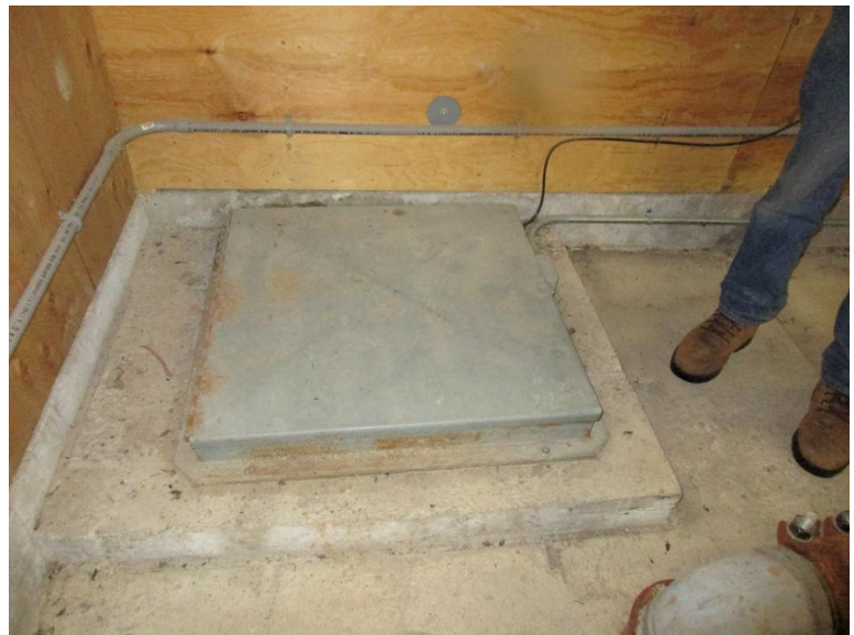
Photograph 10: Storage tank hatch inside pump house
