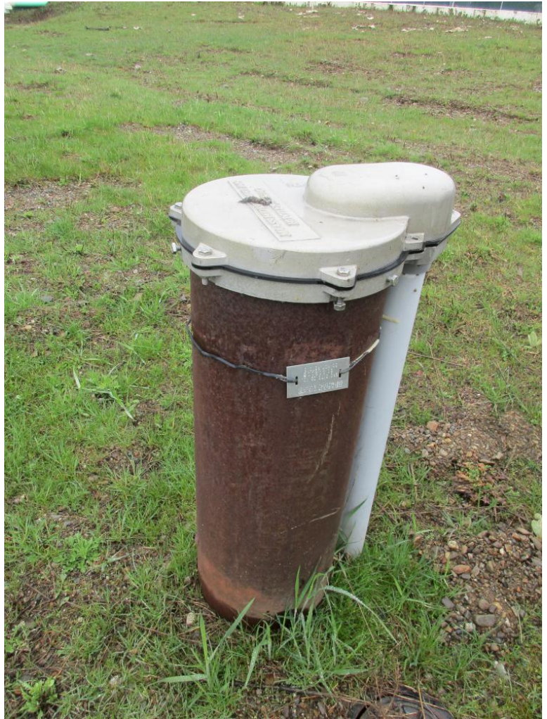
Photograph 20: Well 2 located on the fenced storage tank and pump house lot.
