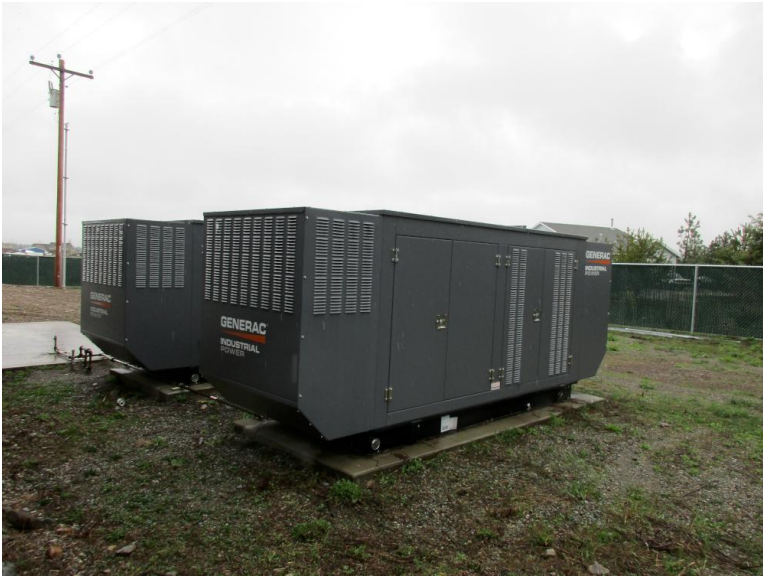
Photograph 1: Two new 150 HP propane powered generators
